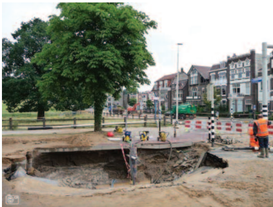
Figure 1 A wash-out pit as a result of a pipe burst can cause severe disruption
